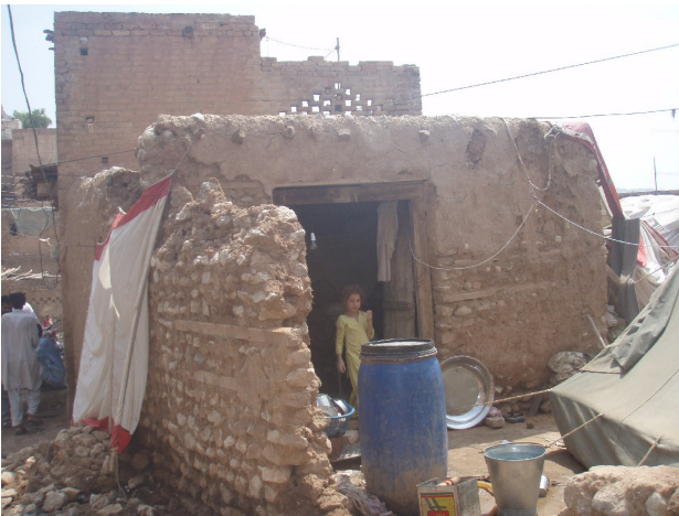
Many houses in Mianwali district have been badly damaged by the rain (UNHCR)
